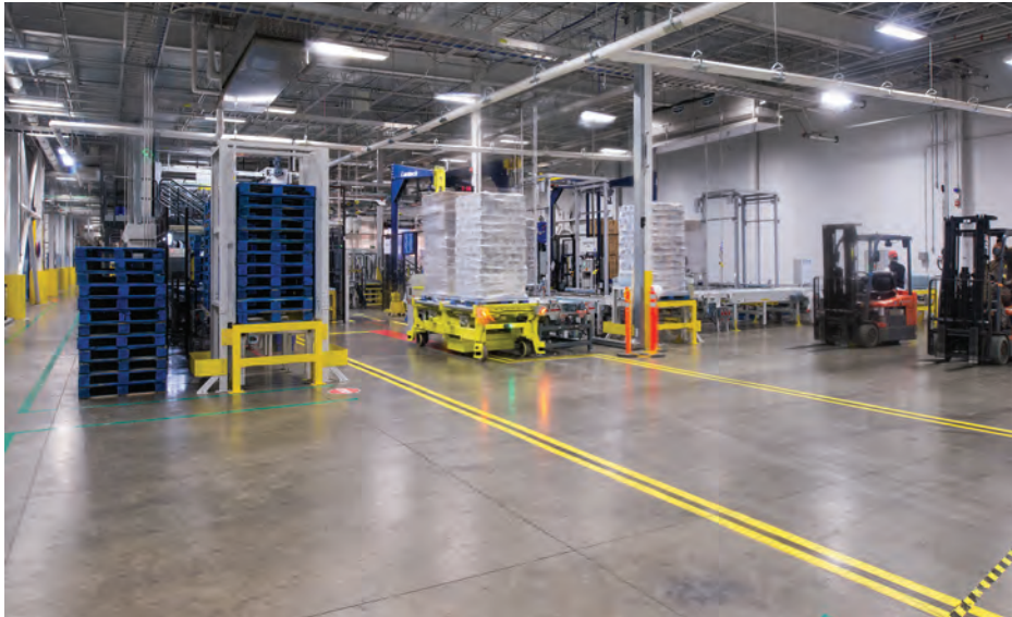
Primus upgraded the baseline lighting to LED lighting with motion sensors at the U.S. Cold Storage (USCS) facility in Covington, Tennessee. This increases light efficiency and reduces power. (Photo courtesy of Primus Builders.)
